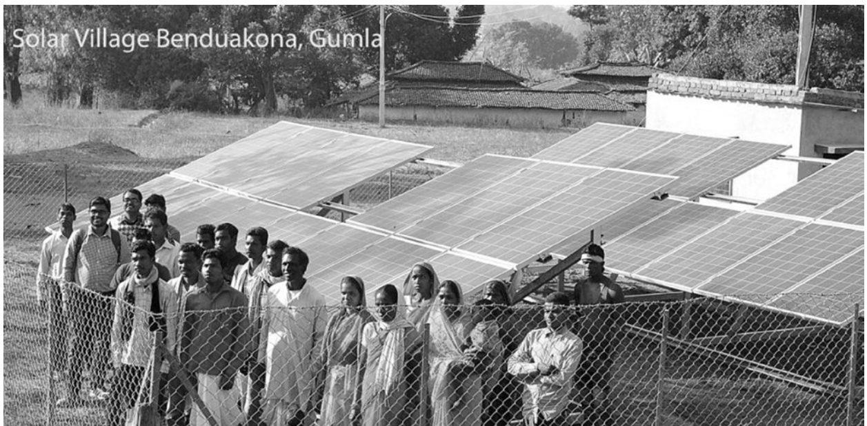
Village Benduakona is now electrified through Solar Grid under the Clean and Renewable Energy Project funded by Bank of America CSR in Gumla district, Jharkhand
