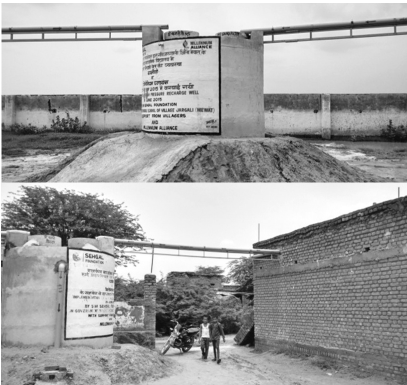
The cylindrical tank built over the ground to collect the water from the high-pressure recharge well, Government High School, Sukhpuri, Nagina block
